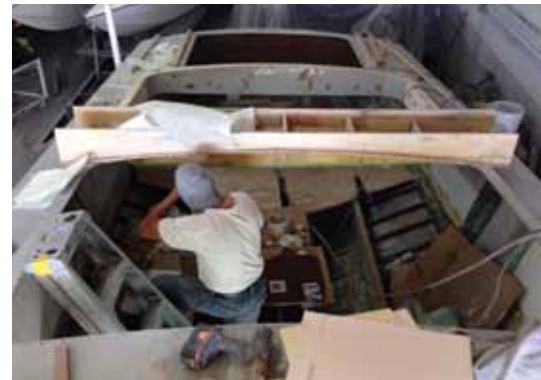
THE BOAT'S deck was rebuilt to match her original layout configuration, and the team removed a walkway from the helm to a forward cockpit that a past owner made.
