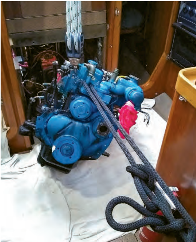
The oily mess of the old engine is pulled up and forward as it's extracted from the engine compartment.
